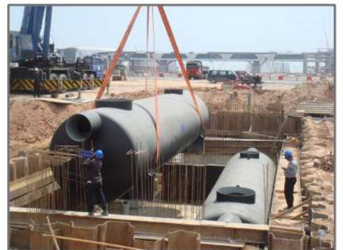
10 off Oil Separator sites for flow rates from 1,368cu.m/hr to 9,900cu.m/hr Malaysian Airports Terminal 2
